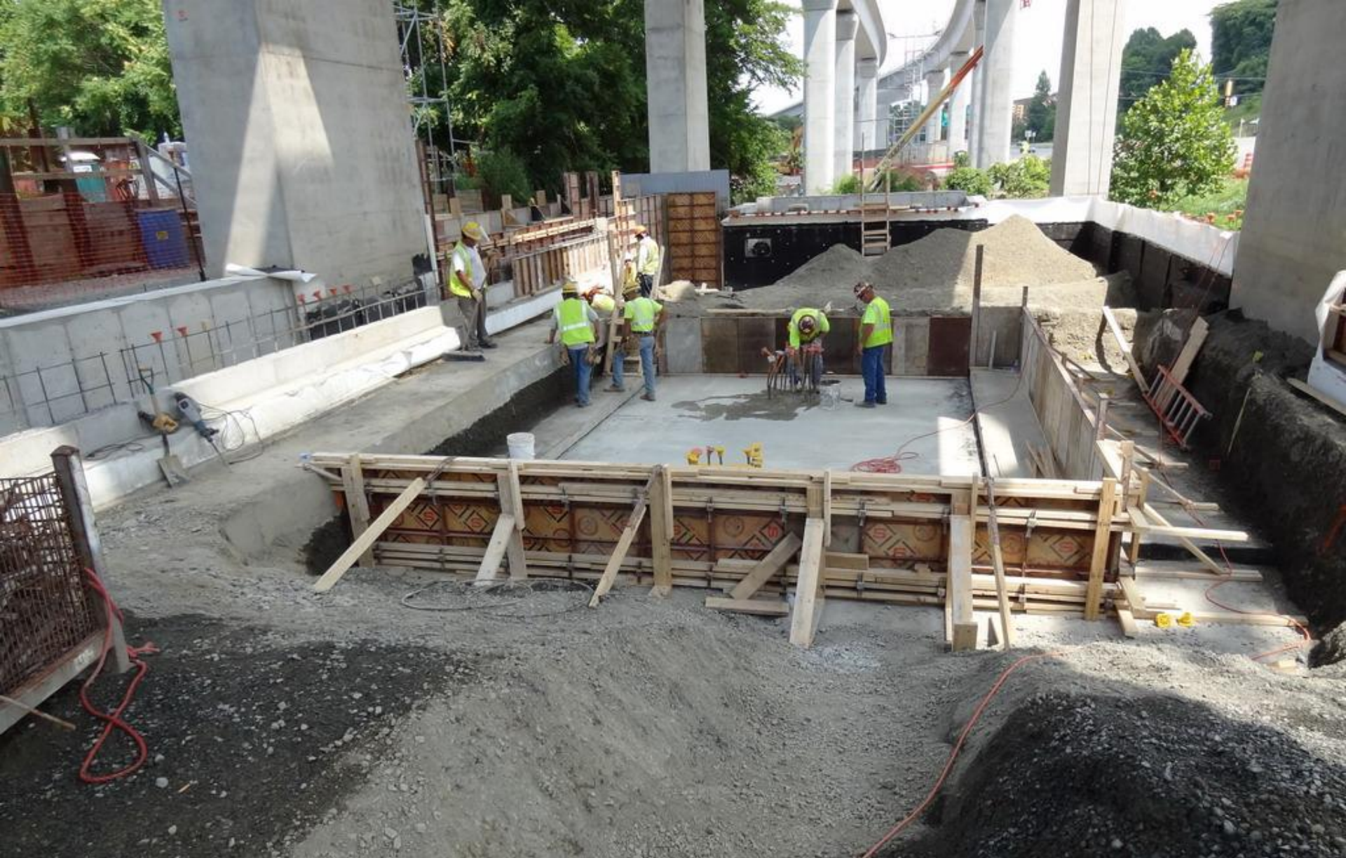
Date & Time: 8/17/2011 1:18 P.M. Location: Rte 123 SB Sta. 655+35+/- @ P-31 IB/OB. Description: DTP Civil forming for Escalator Foundation. Direction: North-East Photographer: CAF-DB-000674-A.
