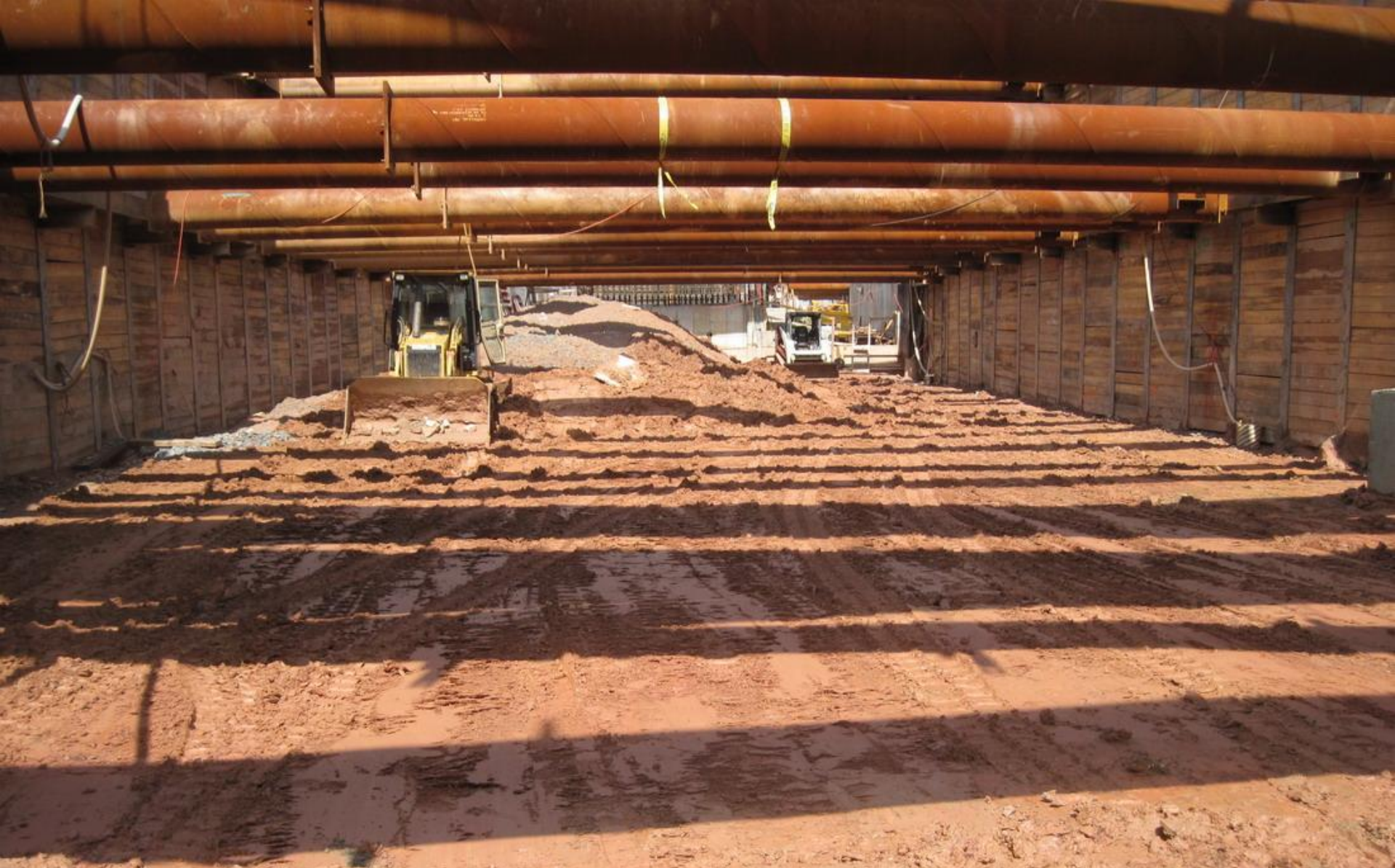
Location: West C&C Tunnel - Stage 2A Looking: West @ OB Unit 7252 Description: Subgrade soil ammended to air out water. Photographer: NTW-DB-001226
